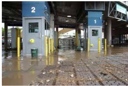
Flooding at Primary Booths
